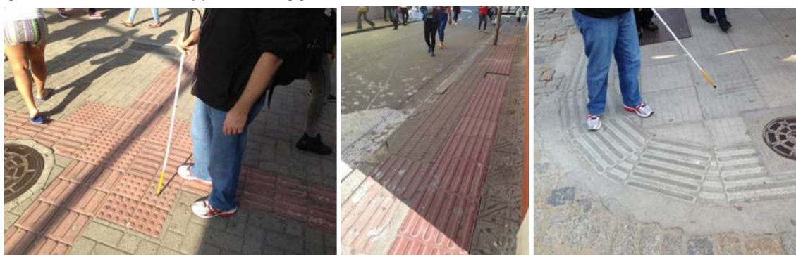
Figure 13 - Tactile floor applied wrongly
