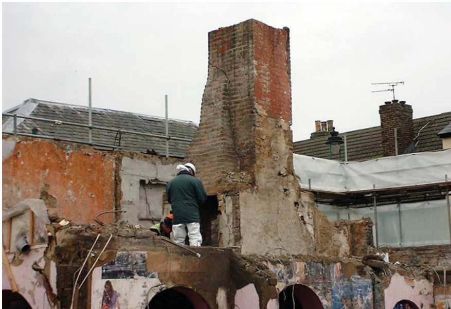
Figure 8 – Demolition of a fireplace and chimney; many items from the Sittingbourne Cache were found alongside the stepped, brick chimney flue. Photo credit: Alan Abbey and Phil Talbot.
