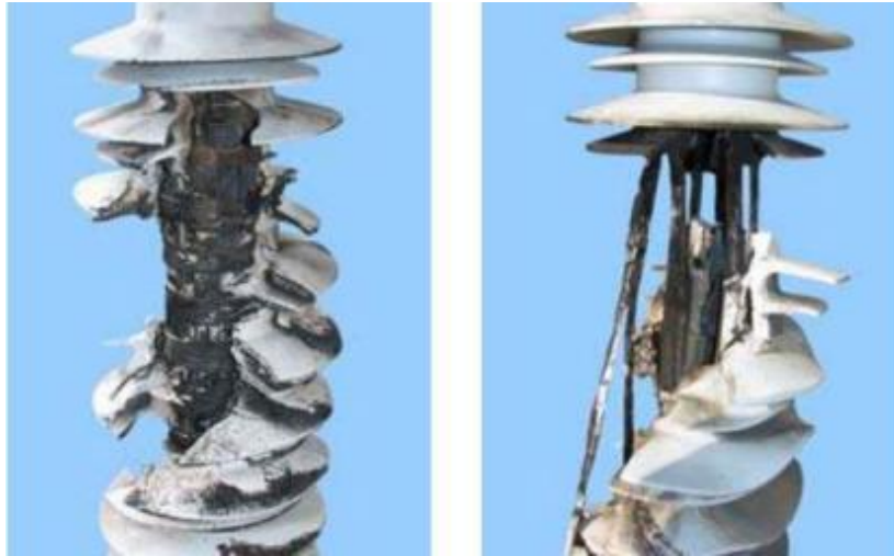
Figure 3. Surge arrester damaged after failure in operation [19].
