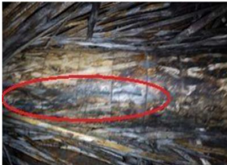
Figure 4. Damage caused by lightning [21].
