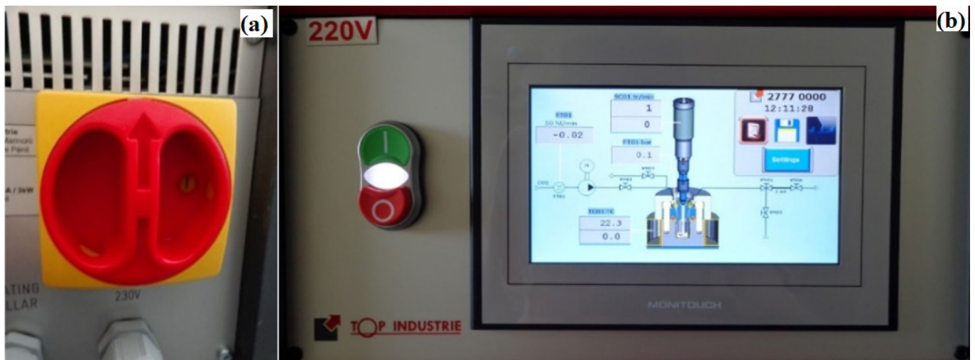
Figure A6. Control cabinet bottom (a) and front part (b).
