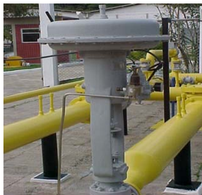
Figura 5 – Pressure Control Valve (PCV).
