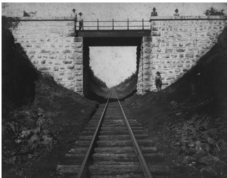
Figure 7. End of the construction of the upper passage in masonry and iron, km 104. Mogiana Company (19??). Unknown author.
