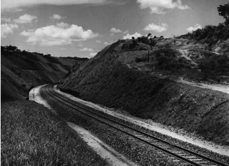
Figure 11: Embankment at Tambaú-Bento Quirino branch line, cutting 35, Km 230. Mogiana Company. Unknown author.
