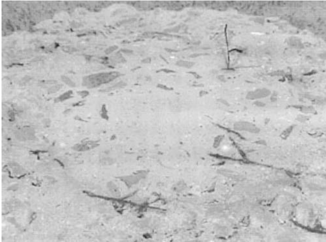
Figure 6: Metal fiber corrosion in RefC|SFco system surface, after humidity exposition.
