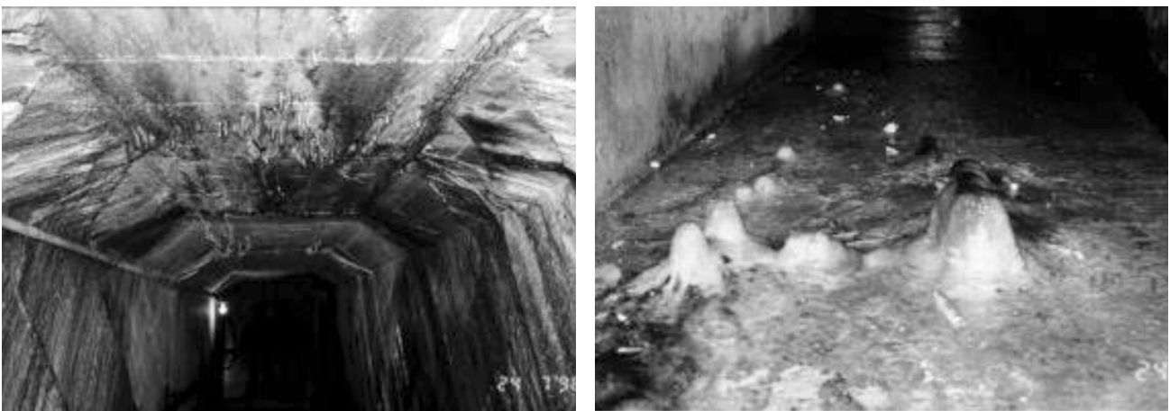
Figure 3: Emerged carbonation as stalactites and stalagmites from concrete cracks in the inspection gallery.
