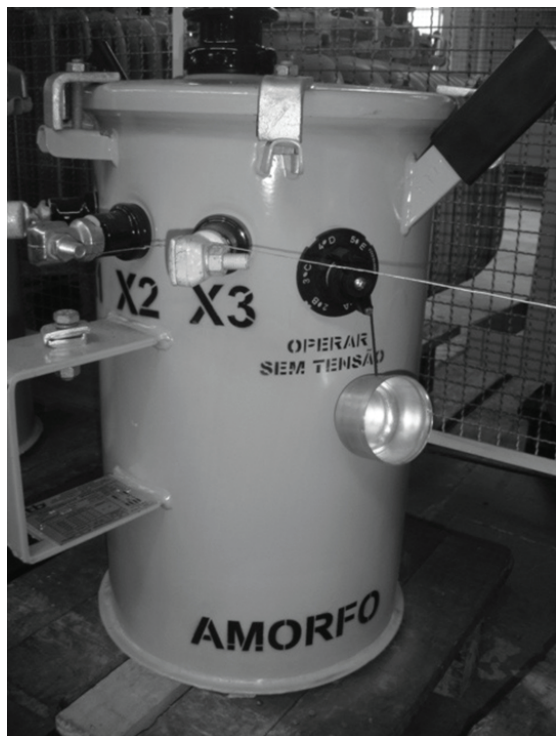
Figure 3. SWER amorphous core transformer with low voltage terminals short-circuited.
