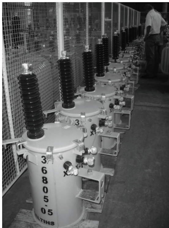
Figure 1. SWER amorphous core transformers in the factory environment.
