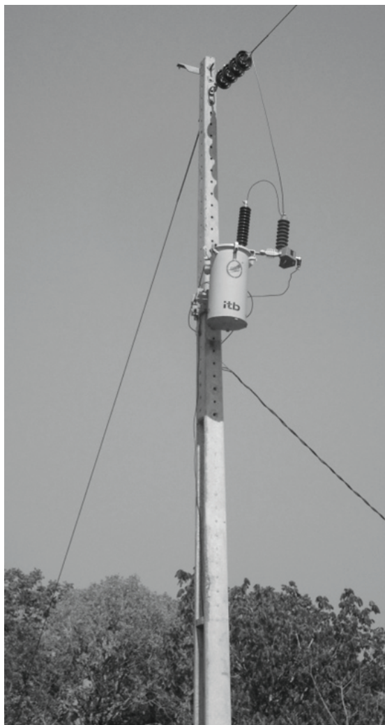
Figure 4. SWER amorphous core transformer installed in the rural zone.
