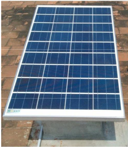
Figure 13. Rooftop solar PV system
