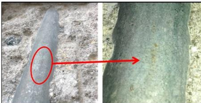
Figure 18: Localized corrosion points.
