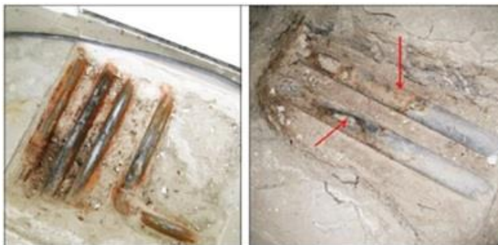
Figure 1: Aspects of external corrosion on galvanized steel pipes.
