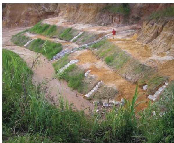
Figure 10: Maintenance work at the rehabilitated area one month after rehabilitation, Sacavém community, São Luís, Brazil. Source: LAGESOLOS, 2008.V
