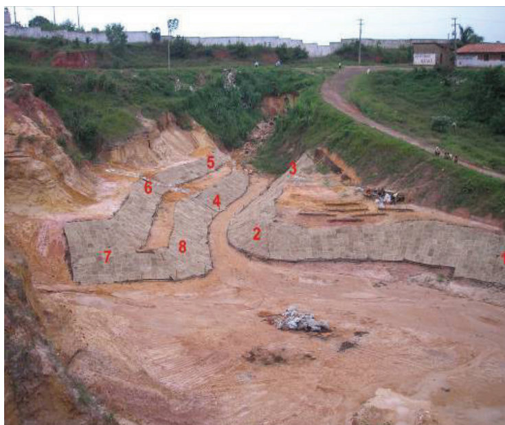
Figure 6: Rehabilitated areas with cover of buriti geotextiles, Sacavém Community, São Luís, Brazil (Areas 1-3 were constructed with men and tractors; areas 4-8 were made in the higher parts with a tractor). Source: LAGESOLOS, 2008.
