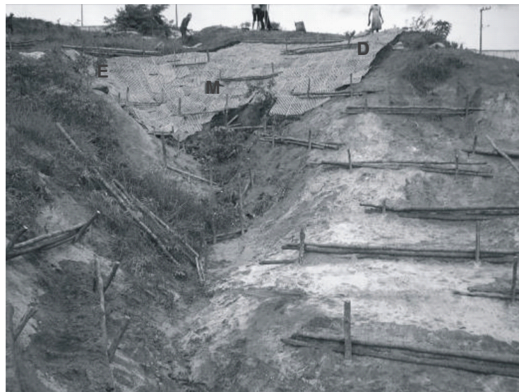
Figure 3: Area 3 of the rehabilitated area, with work in progress. E, M and D were reshaped exclusively by manual labour, São Luís, Brazil. Source: LAGESOLOS, 2008.
