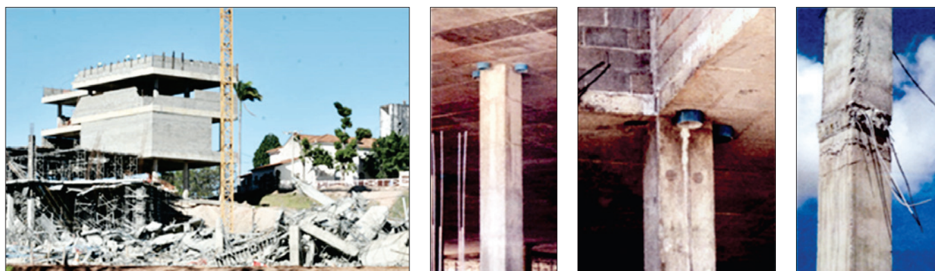
Structure overview post-collapse
