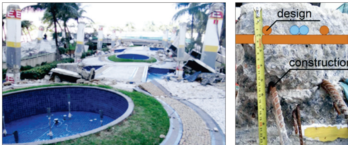
Structure overview post collapse
