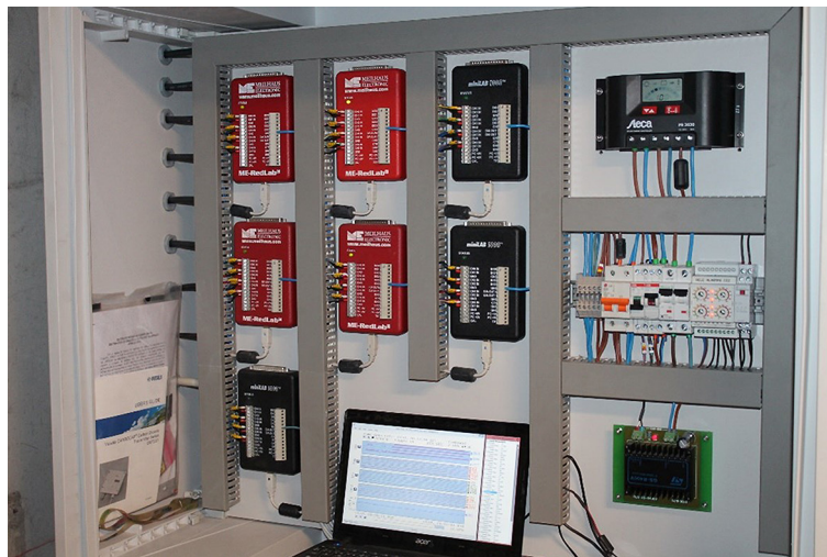
Figure 5 - Monitoring of CO 2 measurement inside the gallery.
