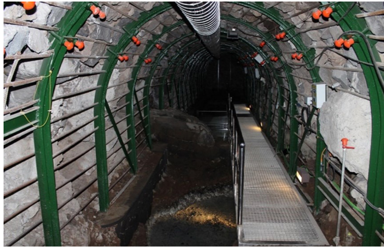
Figure 3 - Interior of the thermal water gallery "Fuente Santa" on the island of La Palma.
