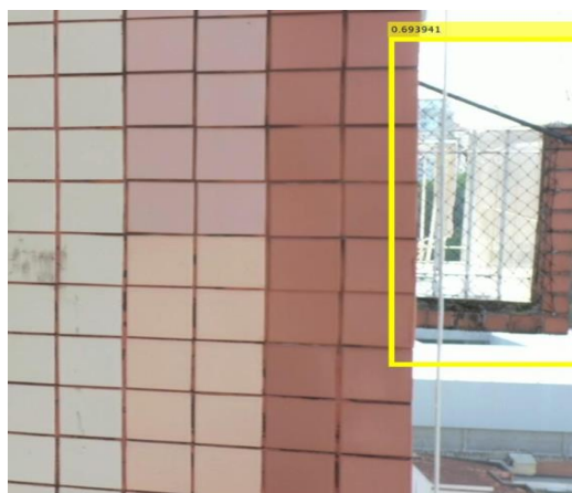
Figure 11 - Guardrail identified as cladding detachment
