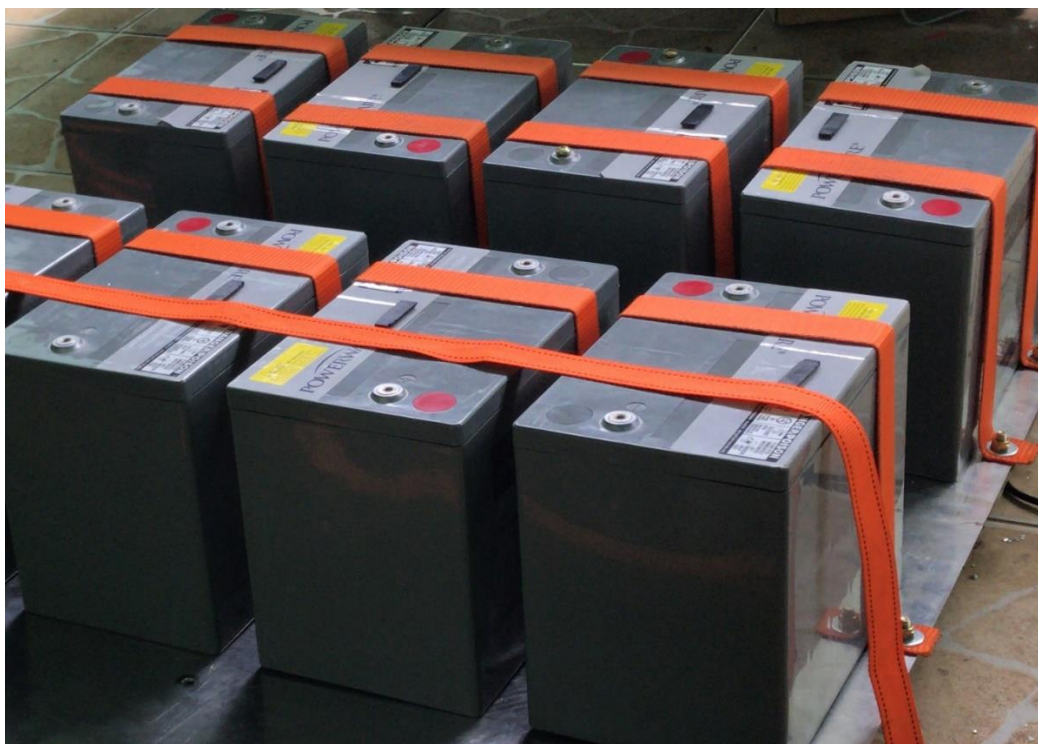
Figure 7. 10.8 kWh battery bank.
