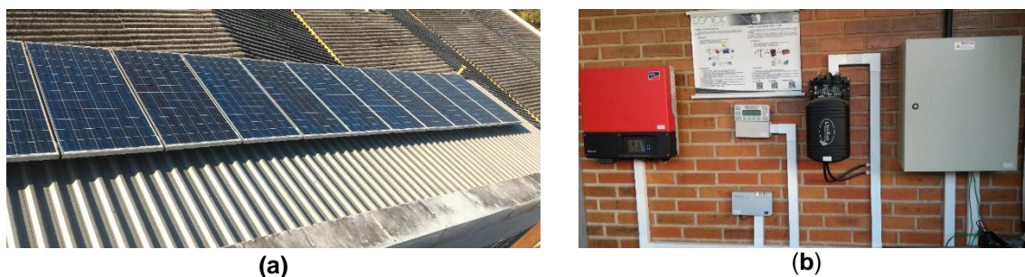
Figure 2. Photovoltaic system at the Federal University of Paraná a) Photovoltaic array; b) Inverter, battery charge controller and monitoring system.
