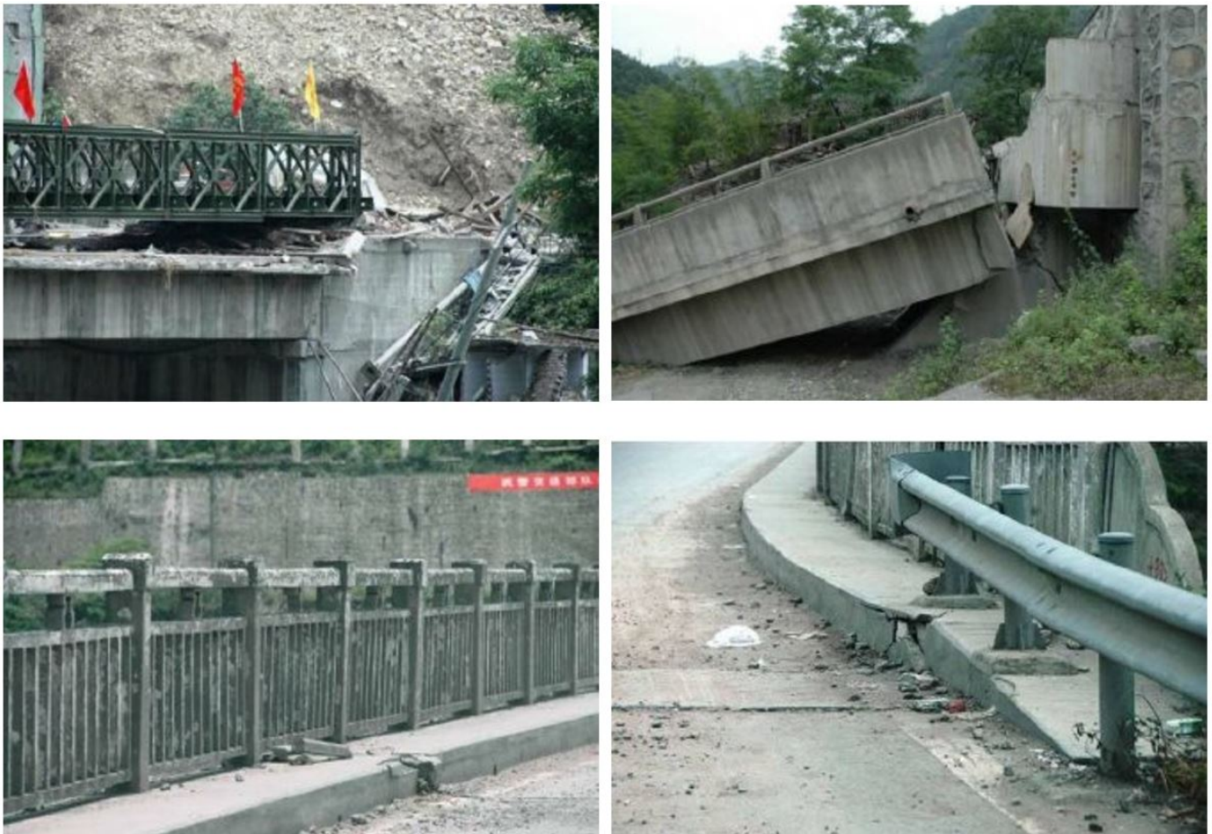
Fig. 2 Damaged expansion joints and their effects on the substructure [6]
