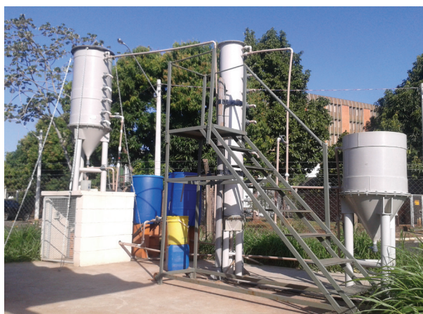
Fig. 1: pilot combined system of wastewater treatment: sewage reservoir (blue tank); from left to right: anaerobic/anoxic filter (AAF) followed by aerated submerged biofilter (ASB) and decanter (DEC) located at the Biological Process Laboratory in University of Campinas (Campinas, São Paulo, Brazil).
