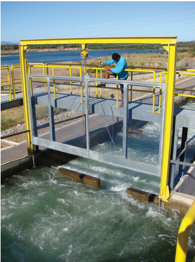
Fig. 1. Screen used to block fish passage through the ladder at Peixe Angical Dam. In this picture, the screen is shown in lifted position (before the beginning of the study).
