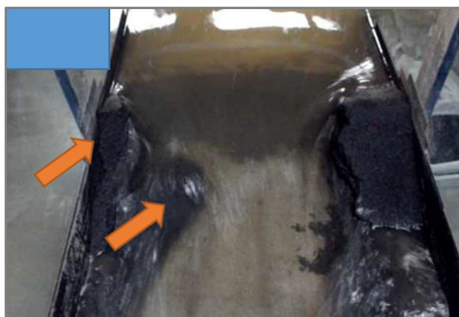
Figure 15. Detachment of parts of left crest and progressive removal of material from the slopes – time 3':56".
