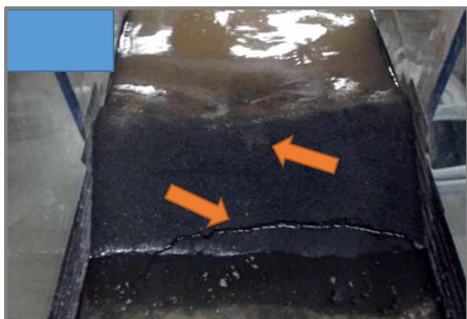
Figure 9. Start of displacement in the low part of the downstream slope simultaneously to the overtopping – time 3':30\".
