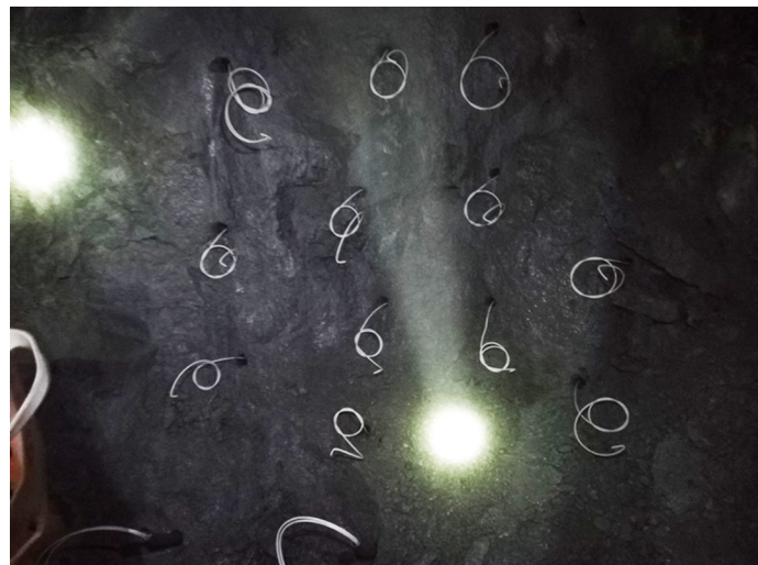
Figure 4 - Blast face, loaded and primed with fire cap and safety fuse, ready to be ignited. Source: Universidad Adolfo Ibañez
