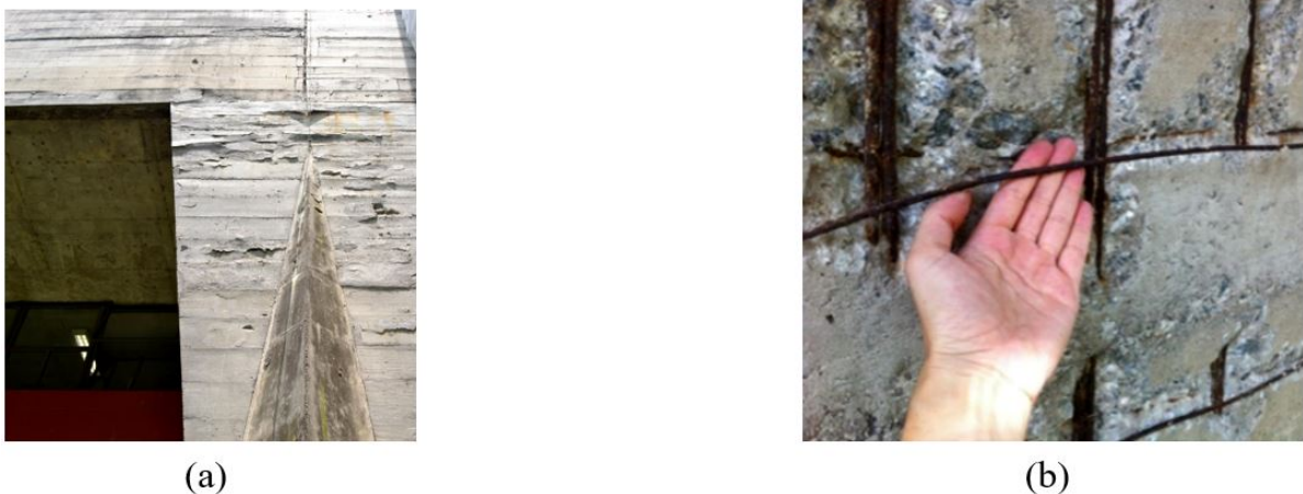
Figure 2. Partial view of NE façade: (a) area with concrete disaggregation on pillar P3 and (b) exposure of corroded reinforcement steel (Photos: authors' collection, 2013).
