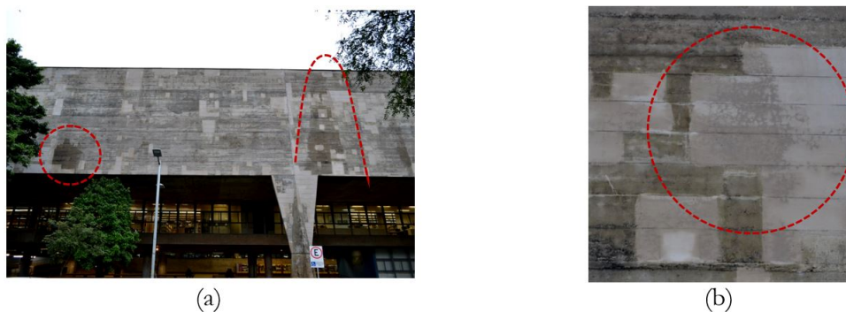
Figure 4. Partial views of SW façade: (a) typical moisture stains and (b) noticeable patch repair cracking after rain water penetration (Photos: Authors’ collection, 2017).
