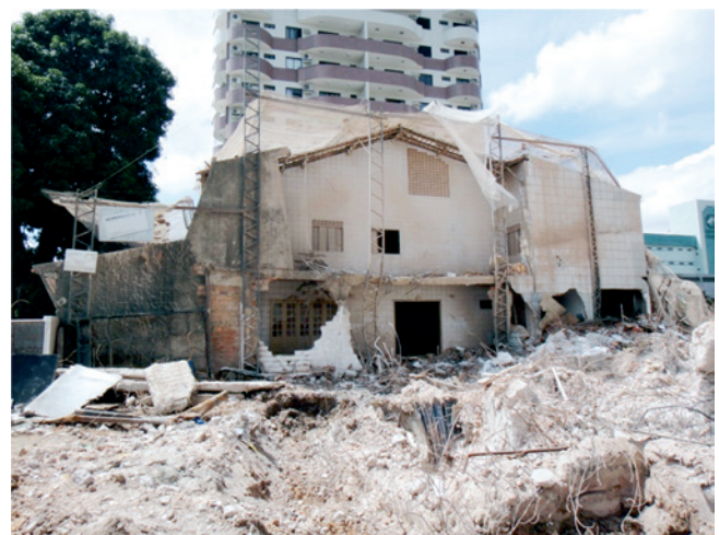
Figure 2 House damaged by the Real Class building debris
