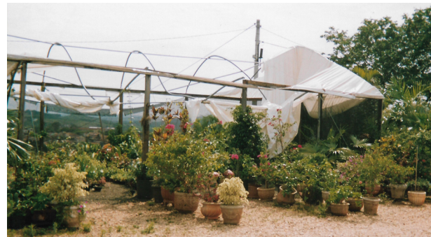
Figure 3 – Single-span greenhouse with the arched roof collapsed by the wind action.
