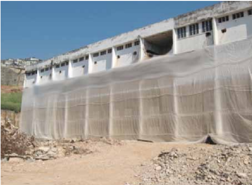
Figure 10 – The Building's last instants. Photo: Alberto Goyena
