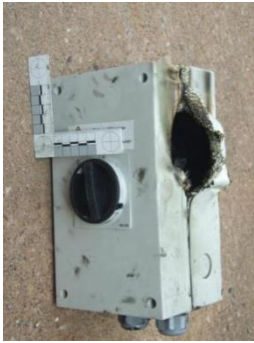
Figure 5 - Switch compartment Source: Adapted. 7
