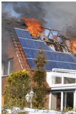
Figure 6 - Fire involving photovoltaic panels Source: Adapted. 7
